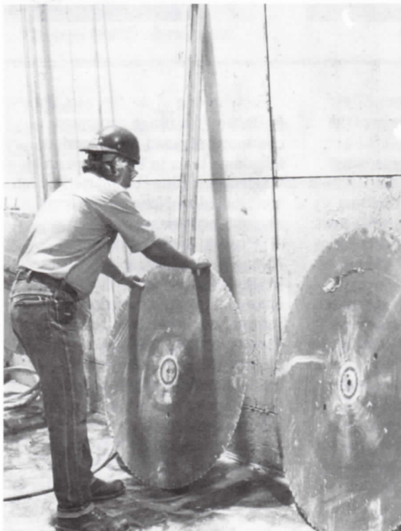
SUPERMAN SHOULD HELP... A contract worker must use oversize saw blades to cut through the irradiation vaults' three-foot thick concrete walls.
