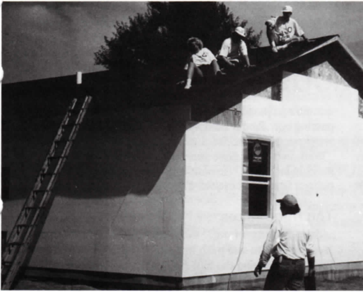
"DON'T TAKE THAT LADDER!"...Would Rick Velasco leave co-workers Patty Ocken (from left), Judy Swanson and Kathy Bernal stranded on the roof? The team from Lucent's Small Business Communications Systems at 110th and O streets worked alongside Omaha Works volunteers.
