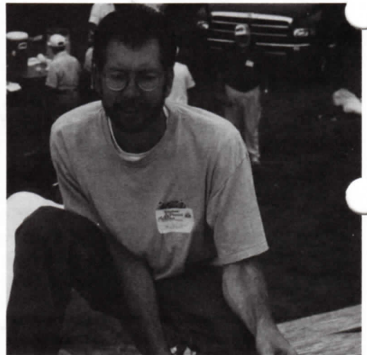
"IF I DON'T LOOK DOWN"...Altitude doesn't seem to bother Robert Wright as he works on the roof.
