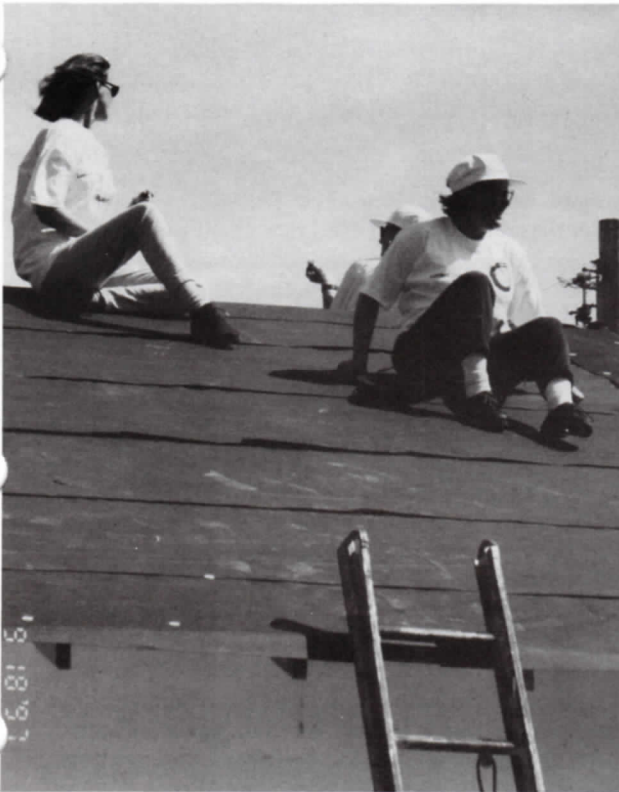
UP ON THE ROOF...Jennifer Huff (left) climbed aboard to help Judy Swanson (forefront) and Kathy Bernal. The Small Business Communications Systems team also helped with the house's telecommunications wiring.
