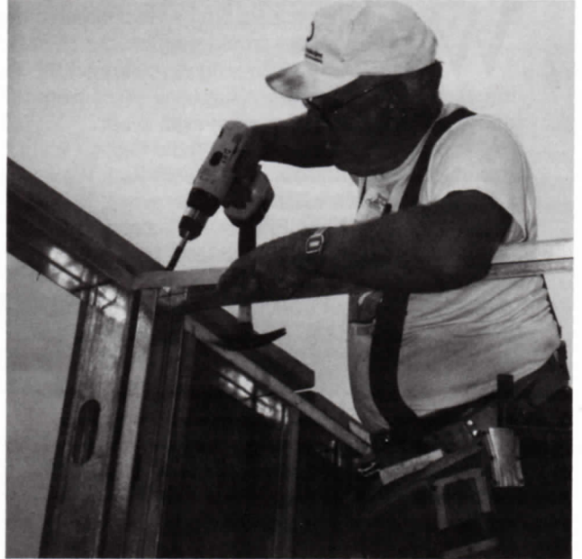
INSERT TAB "A" INTO SLOT "B"...Ralph Brewer drills together some steel studs.
