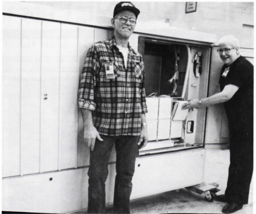
Photo by Linda Ryan IN FINAL ASSEMBLY...Harold Sharp and Karen Hoffmann were responsible for wiring cable to 307 protector blocks in one of the last stages of assembly of the 81C RISLU prototype cabinets.
