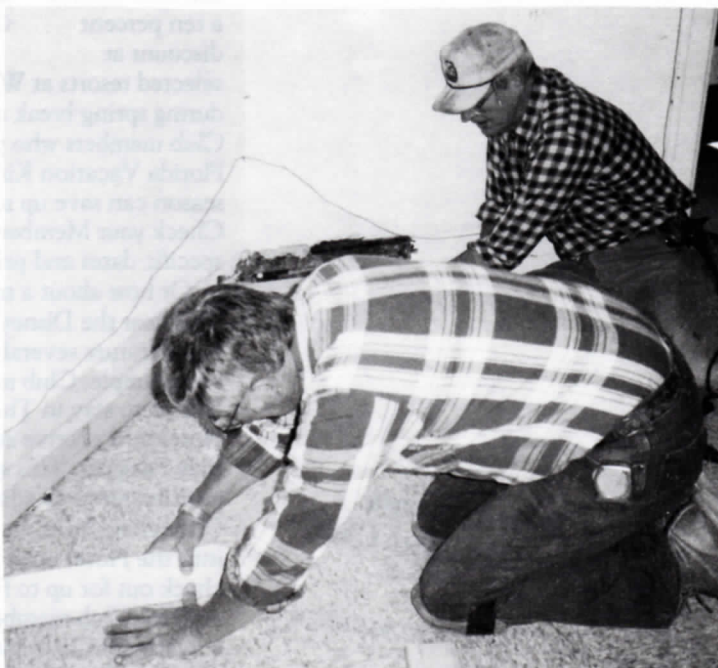
Dewey Ehrenberg (left) and Bob Miller put the finishing touches on a room at the Vincent House. Pioneers have donated over 1,000 hours so far on the project.
