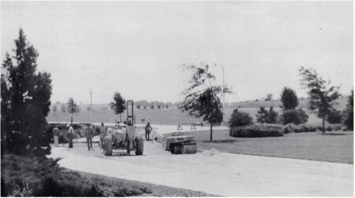
The street in front of the Administration Building was reconstructed to permit more effective drainage.
