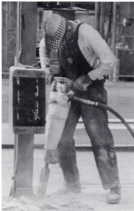
Art Maassen, (244), used an air hammer to break up a concrete pad in order to refinish a portion of the Cable plant floor with creosoted wood blocks.
