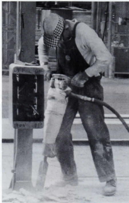
Art Maassen, (244), used an air hammer to break up a concrete pad in order to refinish a portion of the Cable plant floor with creosoted wood blocks.
