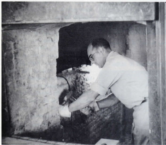
Inside the incinerator, Wallace Williams, (244), repaired the fire brick lining of the destructor chamber.
