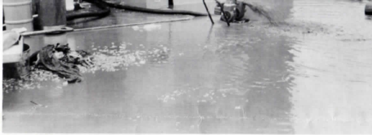
Sewage disposal plant building was flooded and had to be pumped out.
