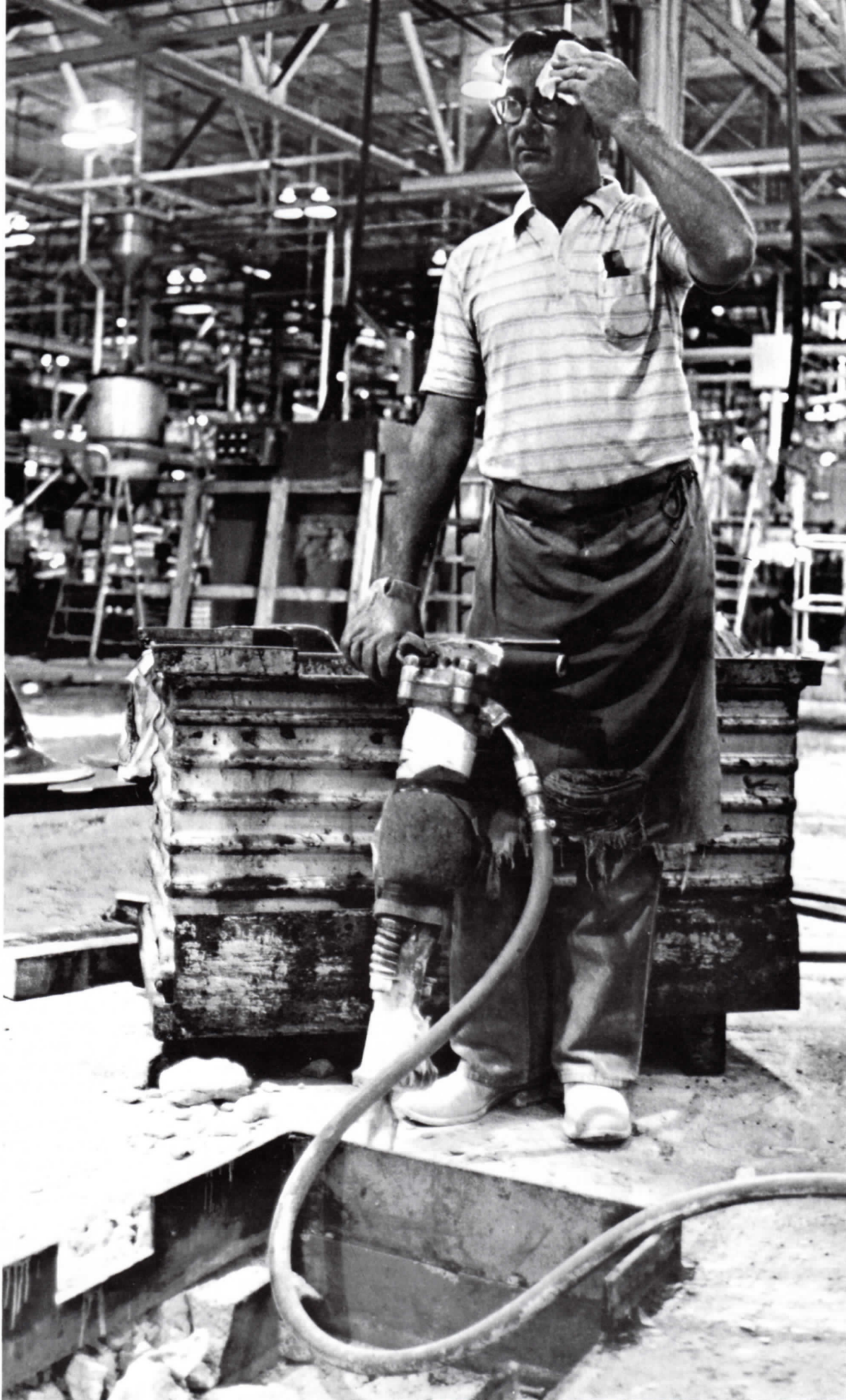
HAMMER AWAY . . . The concrete Duane Suhr is breaking up in the cable shop looks familiar to him. He helped pour it years ago.
