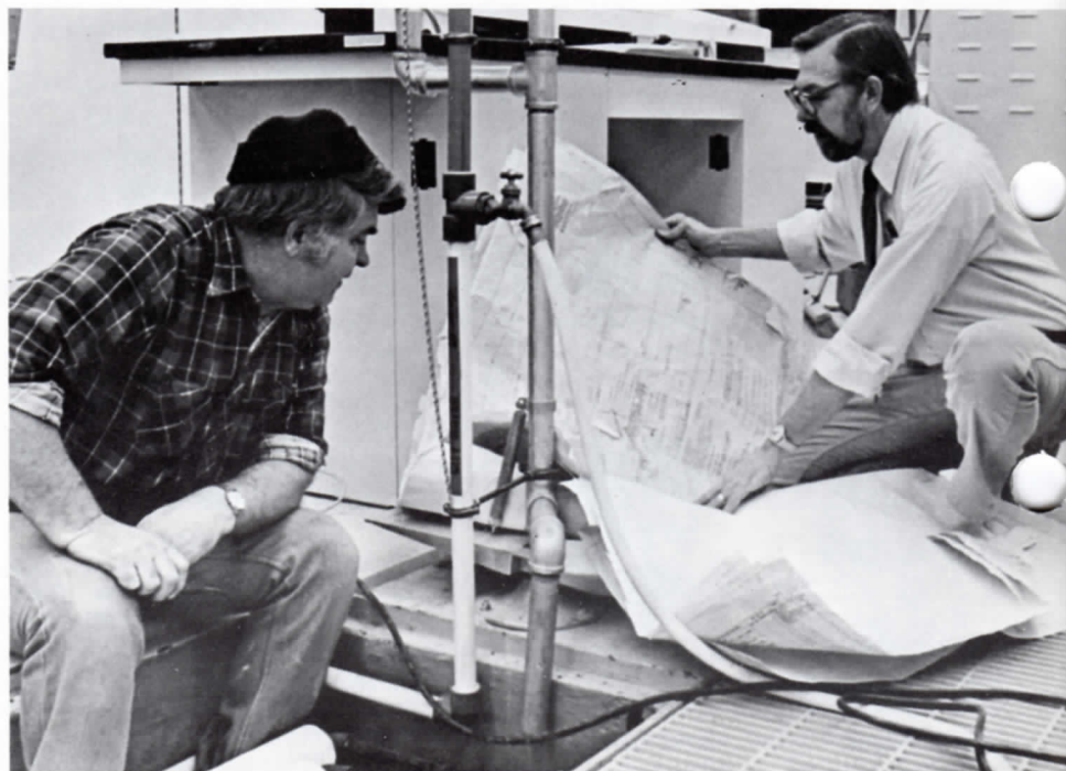
INSTALLATION . . . Senior engineer Chris Christensen (right) of Dept. 731 goes over insulating steam lines and condensate lines with Bill Muckey of Vaughn Insulating. During installation of the platers, Chris was in charge of mechanical engineering while Dick Runnels, also of Dept. 731, took charge of electrical engineering.
