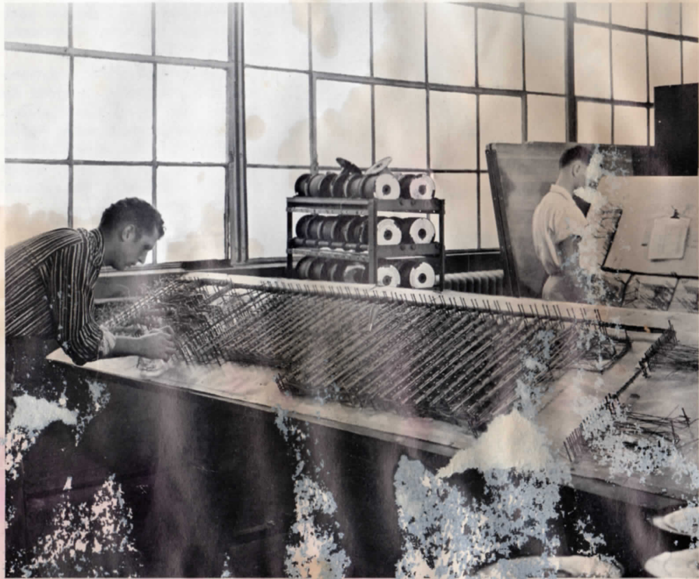
George Ricker and Richard Nielsen work some of the cable forms at the downtown shops.
