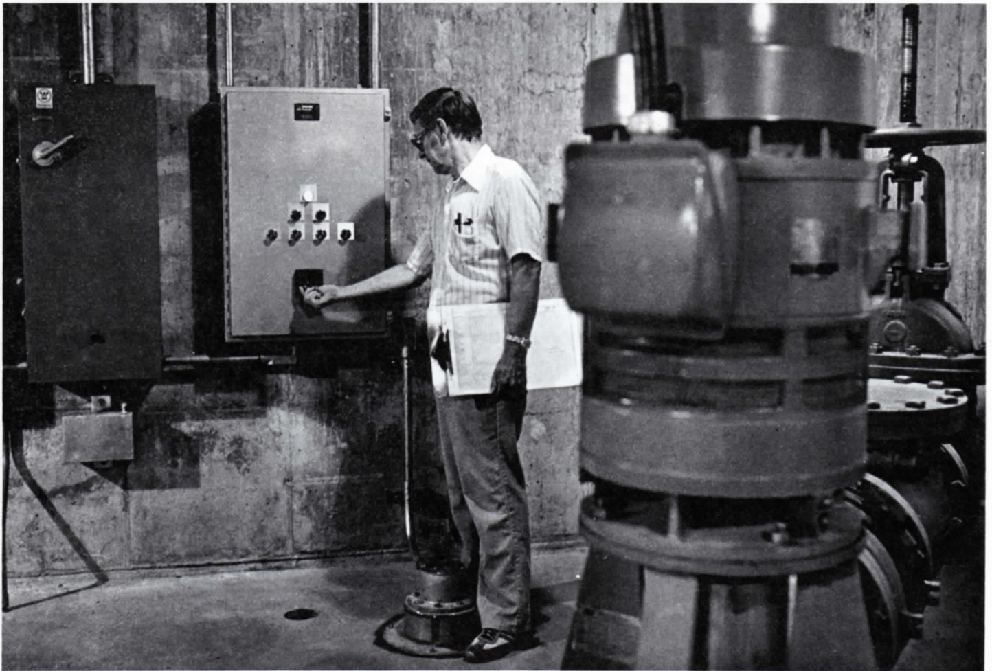
KEEP IT FLOWING . . . Pete Larson, a boiler operator in Dept. 744, monitors the operation of pumps used to send process water to the cooling tower. (One such pump is pictured.) He is standing in the new hot well addition. Warm water to be cooled collects beneath the floor.
